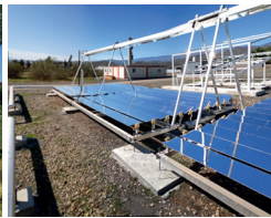
SOLPINTER, Almería (Spain)
